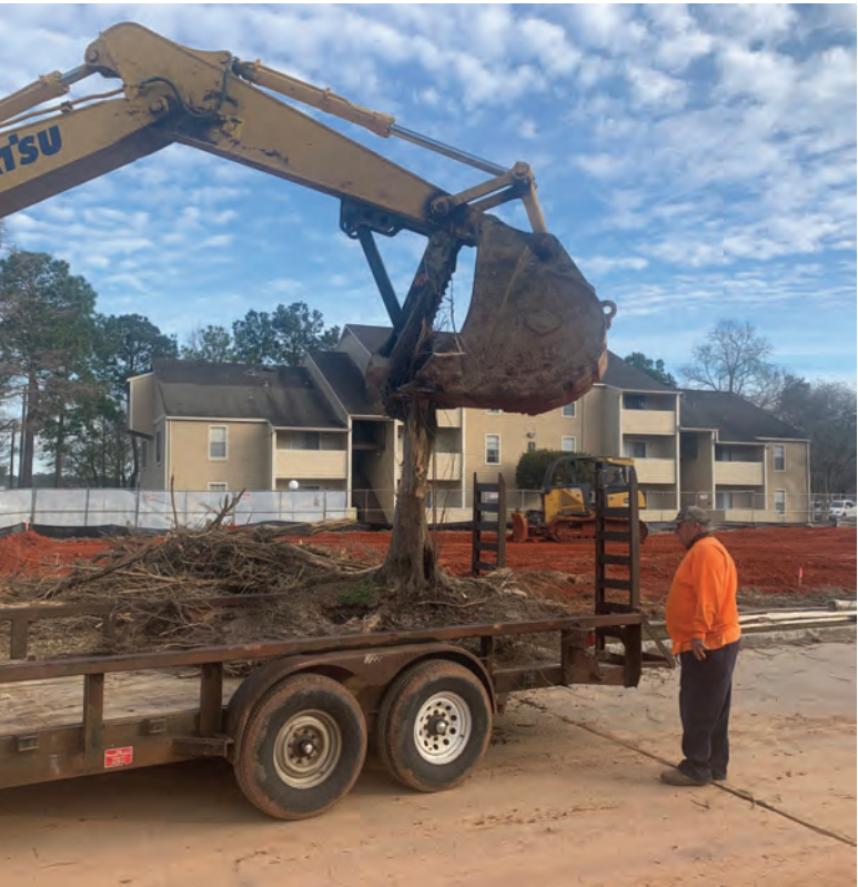
Guy's new acquisition being loaded onto a flatbed trailer by a backhoe
